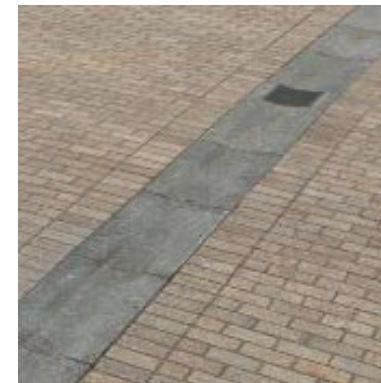
Silver surface drain
